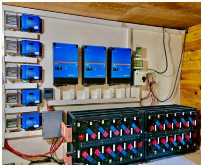
Solar Technical Room
